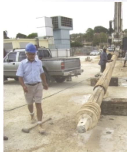
Foundation preparation work for the new low speed diesel engines at Spring Garden Generating Station
