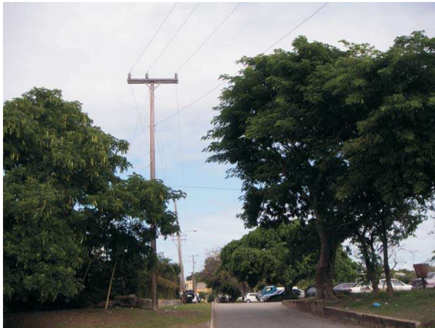
OVERHEAD 24KV POWER LINE
