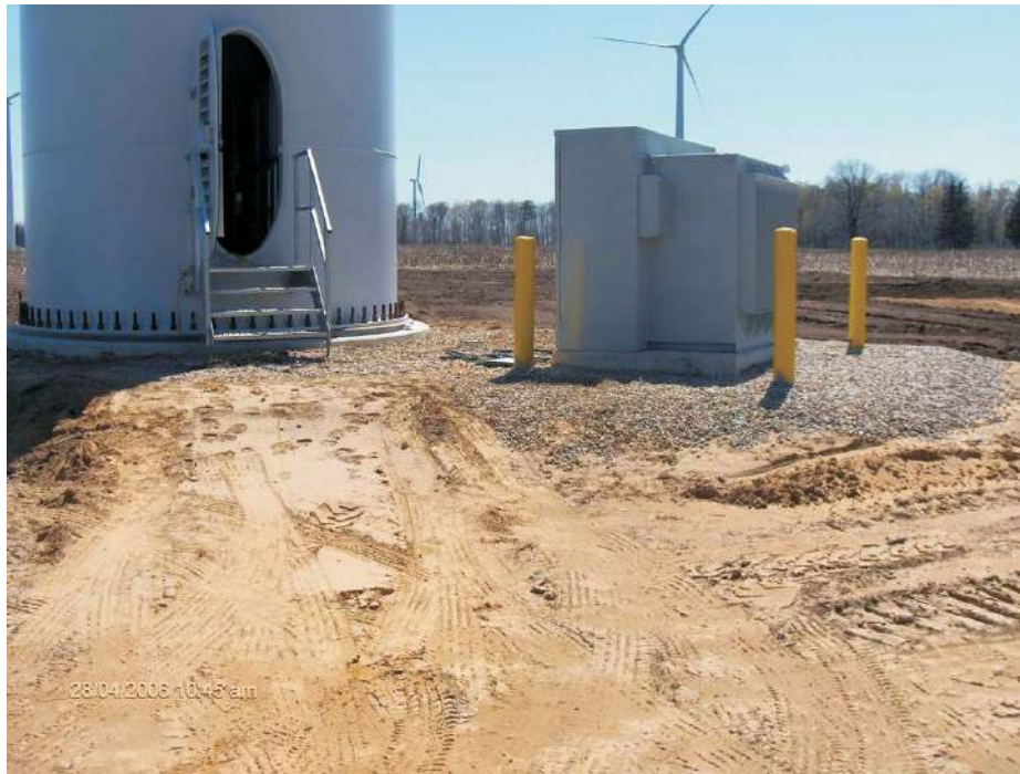
TOWER BASE AND TRANSFORMER
