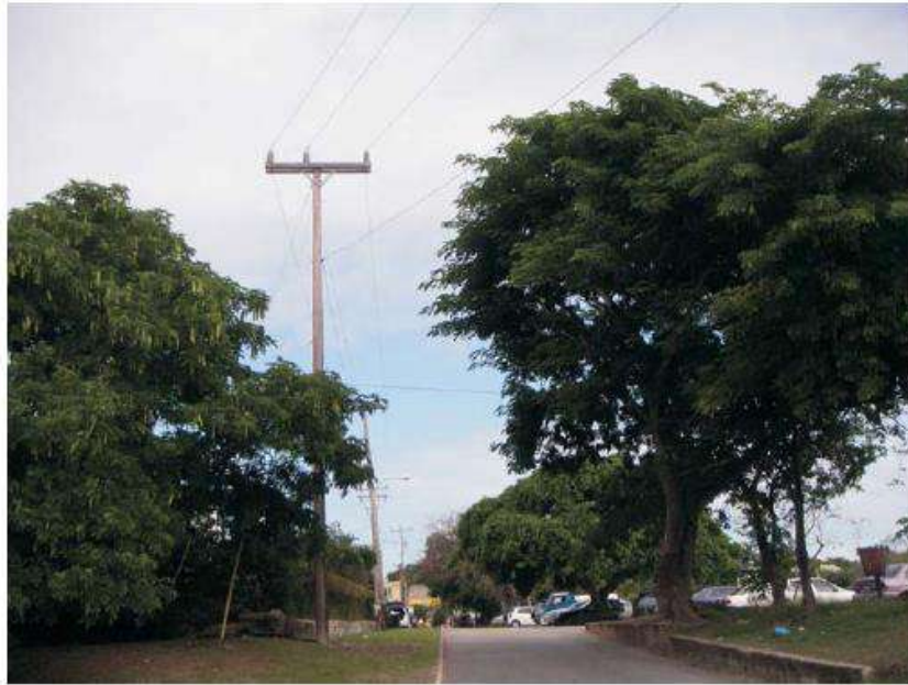
Figure 2-3: Standard Overhead 24 kV Power Line used in Barbados
